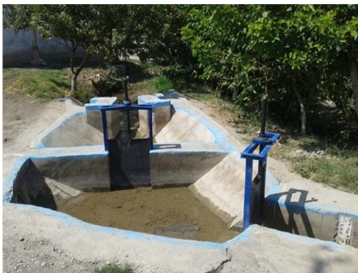
«Kahramon Davlat Sahovati» farm, facility for water supply and measurement
